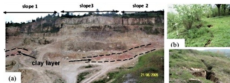
Figure 2 (a) Excavation slopes where landslides occurred and previously developed tension cracks (b).
