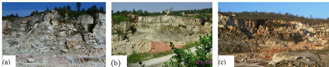
Figure 3. The landslides occurred on 3 October 2005 (a), 20 March 2006 (c) and 19 October 2006 (b) in Araklı- Tasonu Limestone Quarry.
