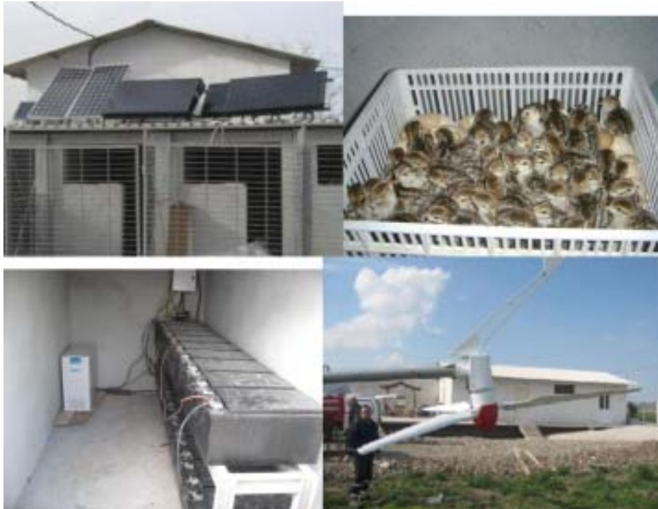
Figure 4 Installation of RE system in Bigadic PF (see online version for colours)
