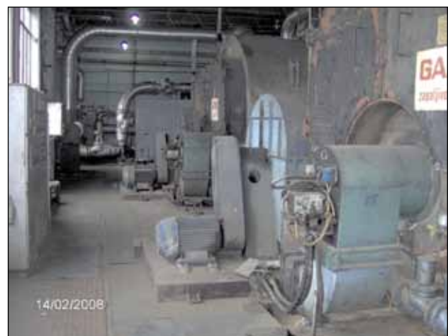
Picture 4. A display of the work place in the boiler-room
