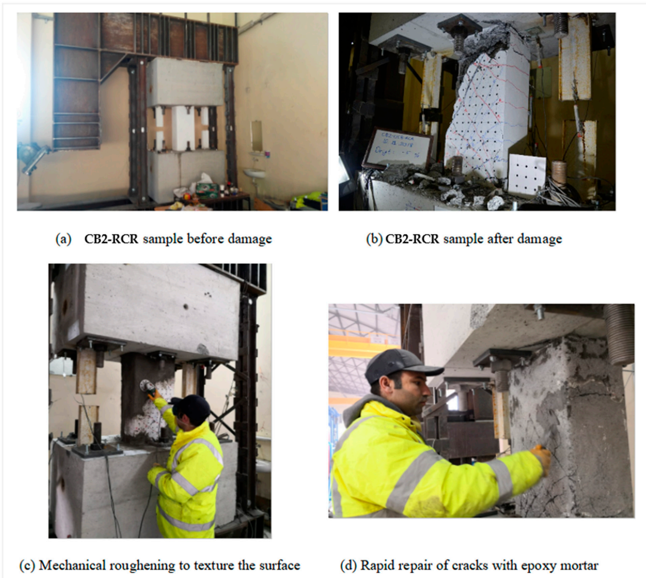
Figure 7. Stages of inflicting earthquake damage and strengthening on the CB-RCR specimen.
