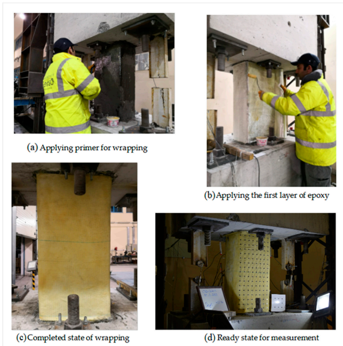
Figure 8. Stages of wrapping the CB2-RCR specimen with GFRP and preparing it for testing.
